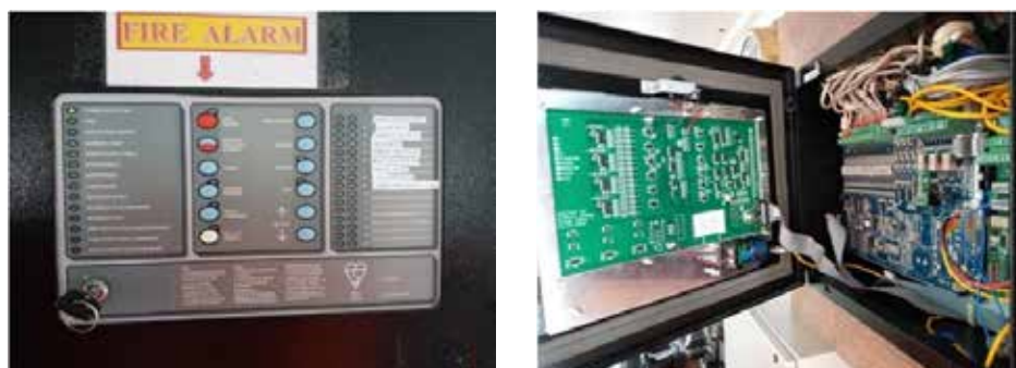
Fig. 2. Disabled audible fire alarm and disconnected cable
