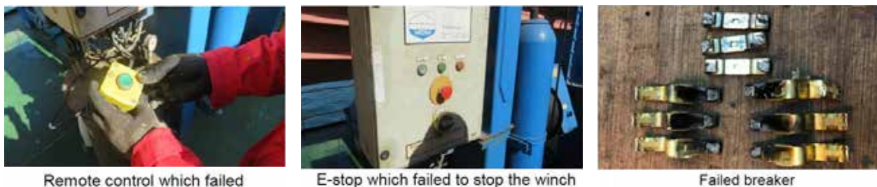
Fig. 1. Remote control, emergency stop and failed breaker
